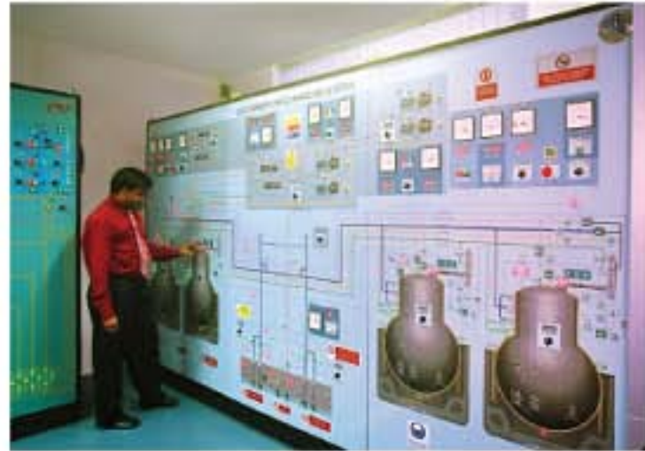
The LNG cargo tank/piping panel on the Anglo Eastern simulator provides an exact replica of the ship
